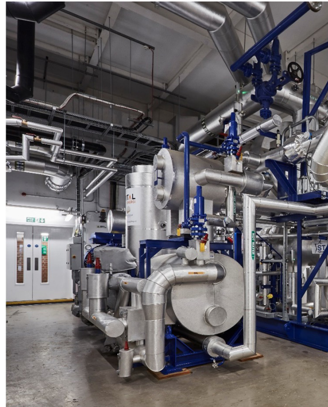
The 2 x 2.65MW Water Source Heat Pumps From Star Renewables.
