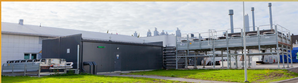
The installation are complete and the modular AmbiHeat – heat pump plant produces Zero Emission heating and cooling for Orion Medical Factory needs.
