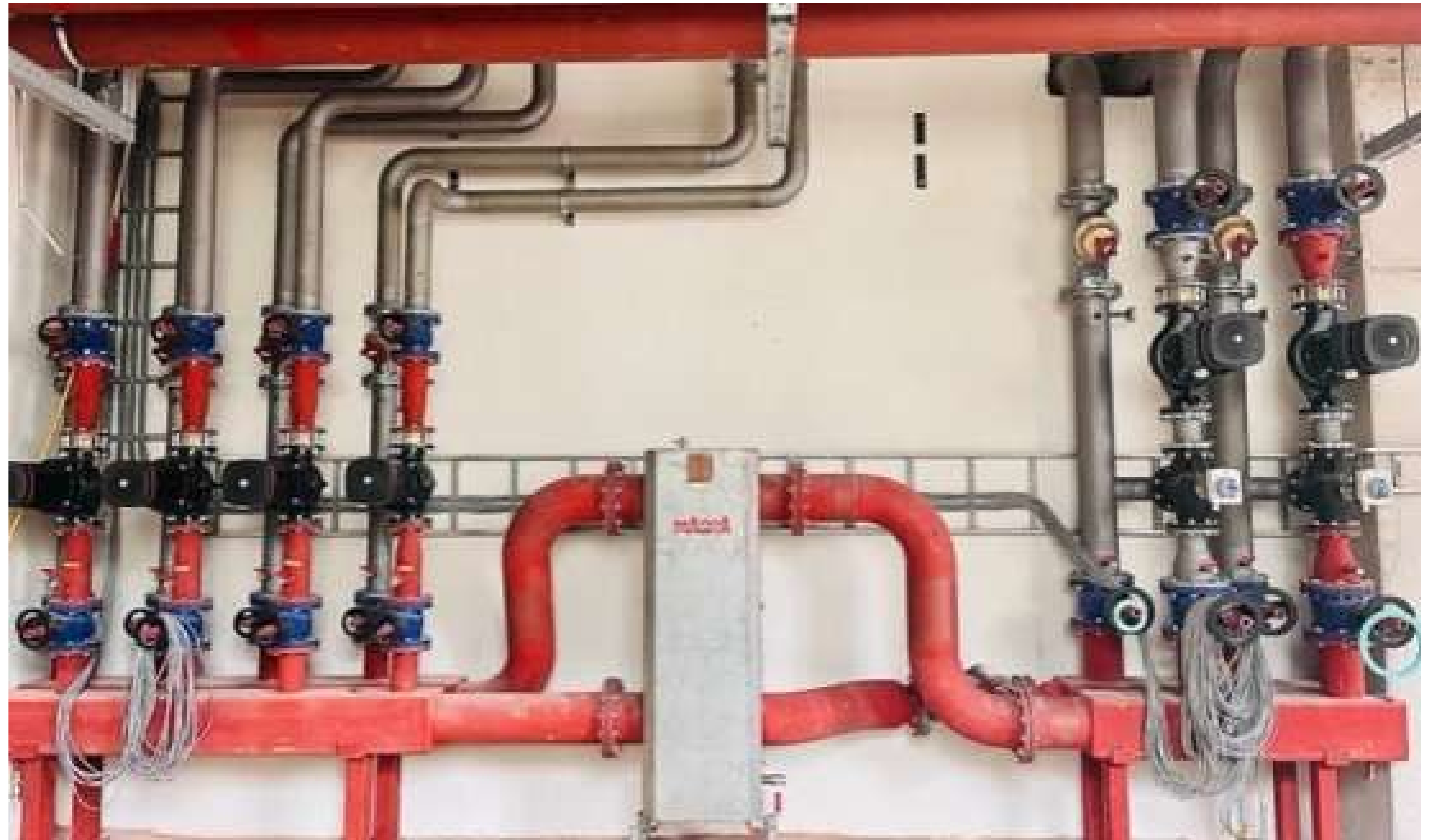
Hydronic installation including de-coupler without insulation - Copyright Daikin Airconditioning Central Europe HandelsgmbH, AHT Cooling Systems GmbH
