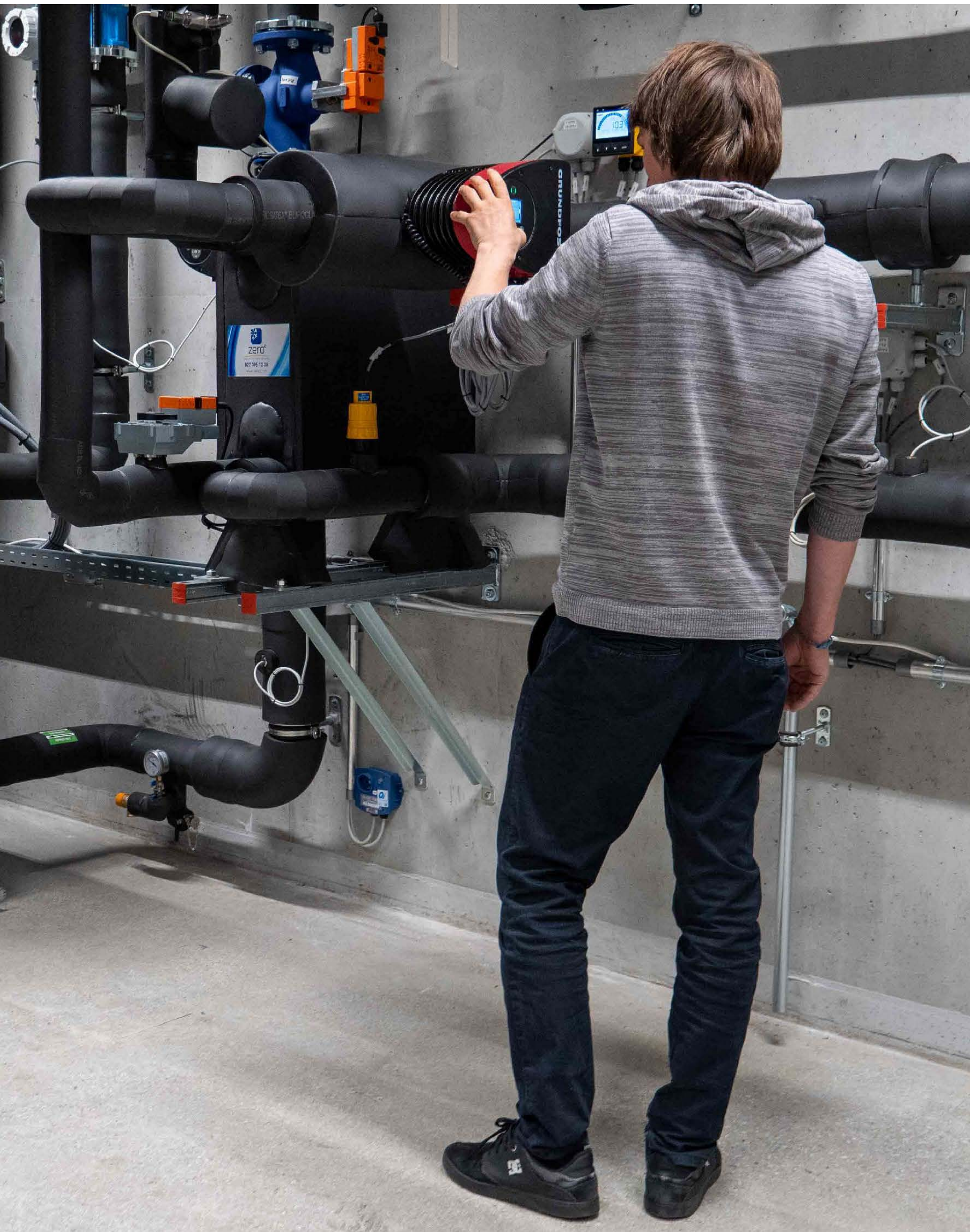
Sion Substation - Copyright ExerGo
